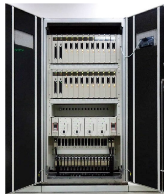
Electronic Terminal Rack
