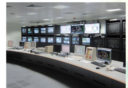
Operation Control Center
