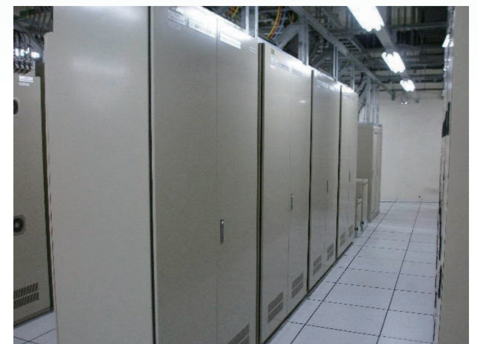
Signaling Equipment Rack
