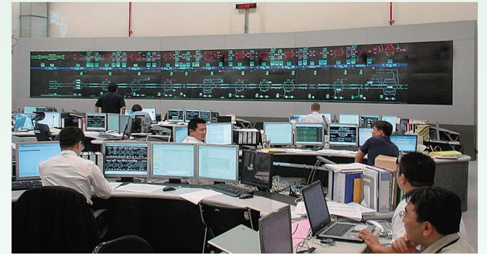
Taoyuan OCC (Operation Control Center)
